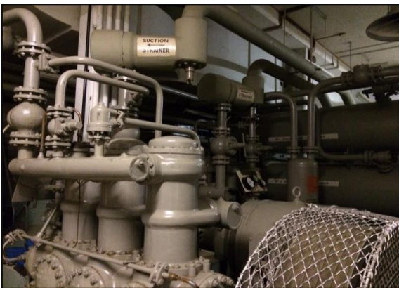
Air Conditioning Plant
